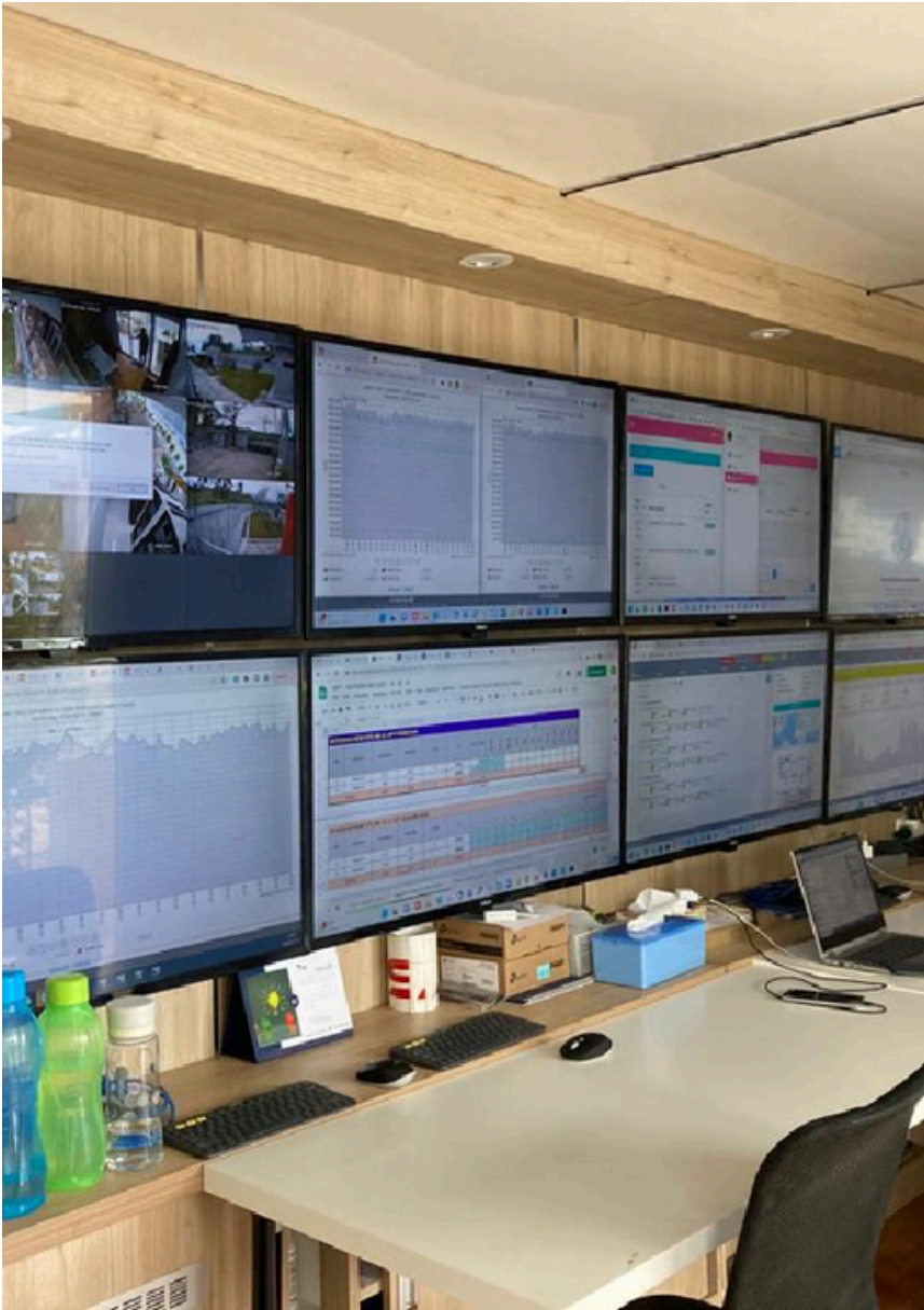
Ruang monitoring NOC
