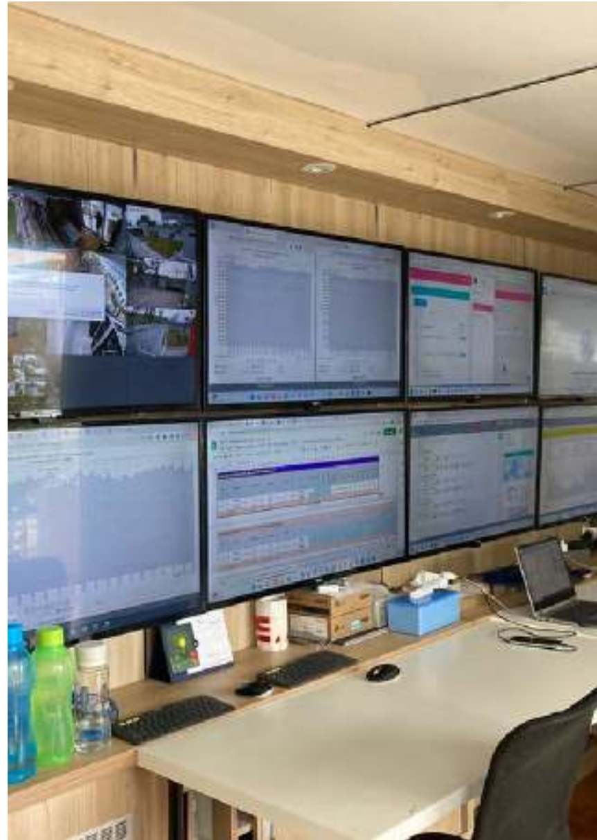
Ruang monitoring NOC
